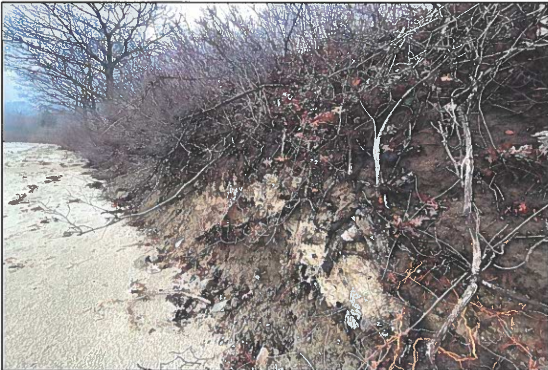
Photograph Two. Facing southwesterly– view of portion of shoreline that is eroding. Riprap will begin at base of slope.
