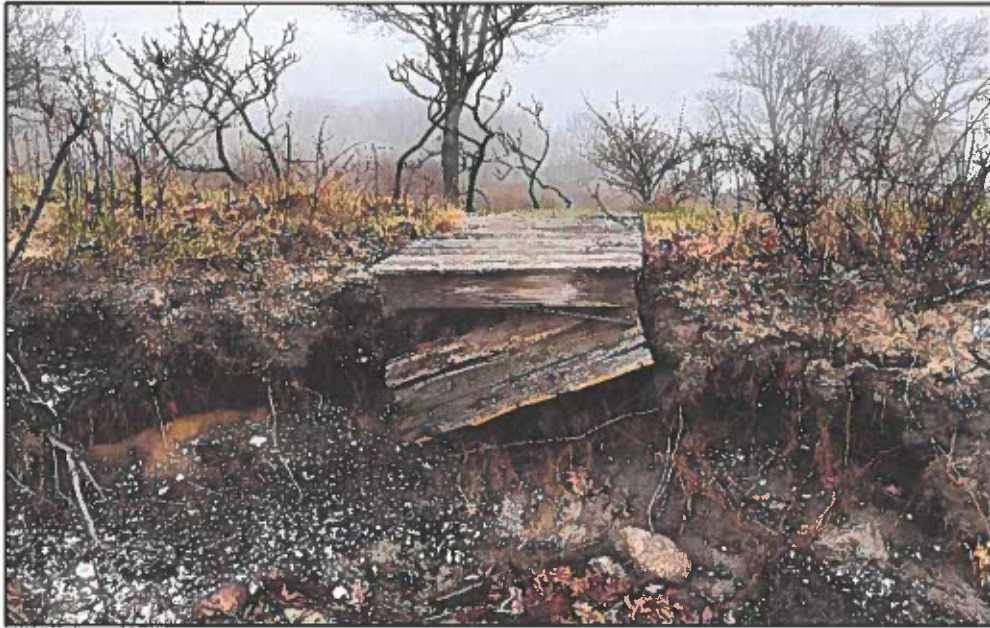
Photograph Five. View of stairs that were destroyed in the 2023 storms. Hardscrabble stairs constructed within the riprap will replace these.
