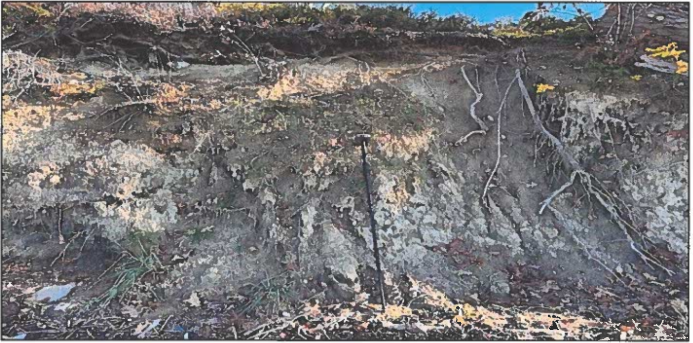
Photograph Eight. Additional view of failing slope. GPS pole pictured is six (6) feet long, for scale.
