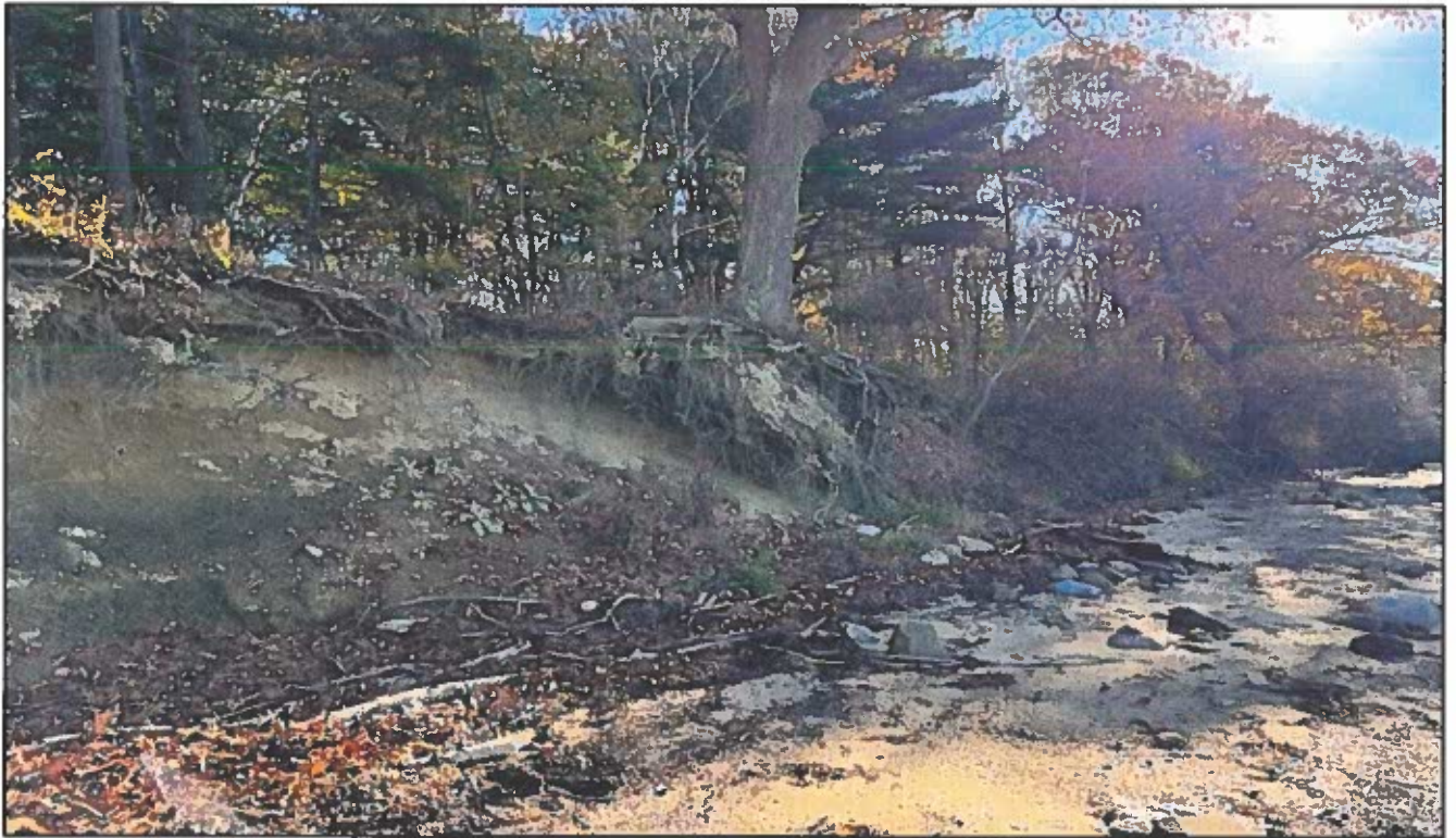
Photograph Five. Additional view of falling bank.
