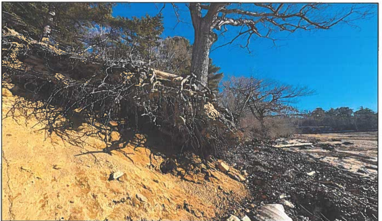
Photograph Four. Additional view of failing slope.
