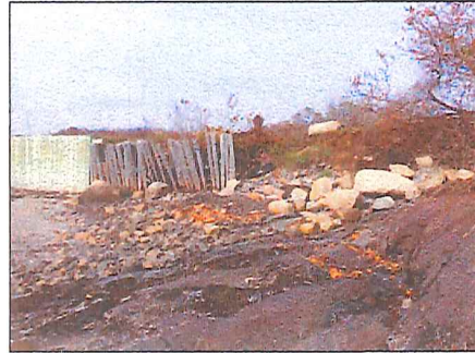
Photo 2 - Bulkhead Section "C" and bank erosion
