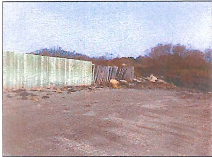
Photo 1 - Bulkhead Sections "B" and "C" and bank erosion
