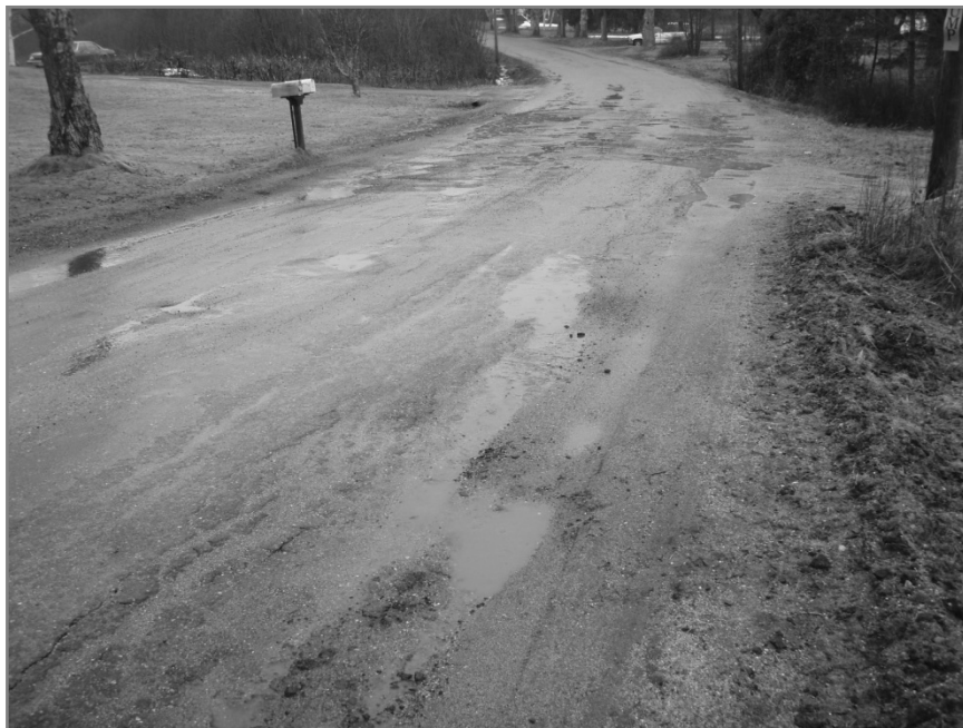
Figure 2 - Drainage, Roughness, Cracking and Potholes on North Road (2009)
